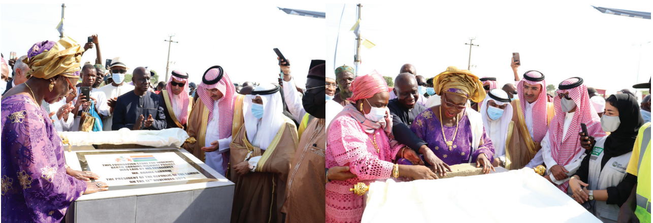
Vice President Dr Isatouray Laying the foundation stone for the expansion of the Bertil Harding Highway
