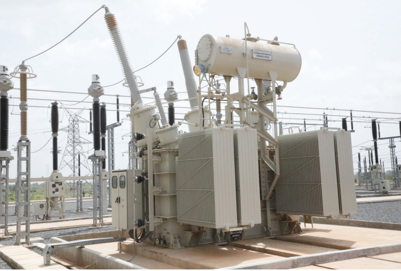
OMVG Substation in Jarra Soma
